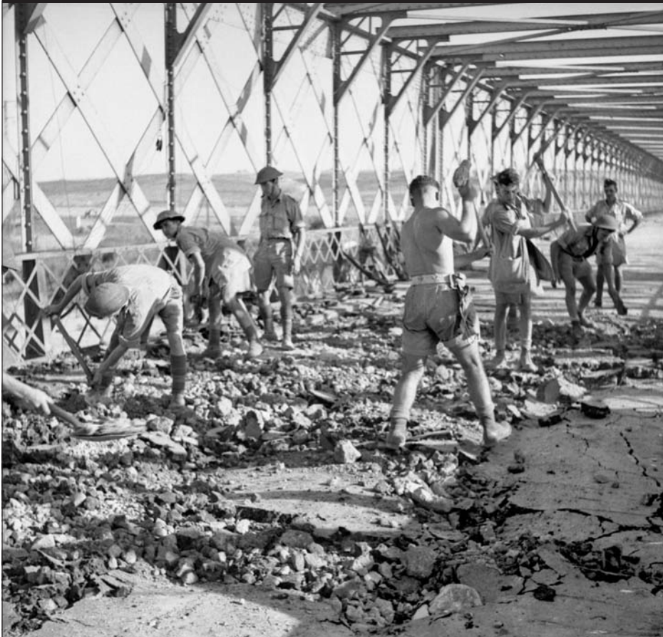
The prize: Royal Engineers repair damage to the bitterly contested, 400-foot-long Primosole Bridge over the Simeto River several weeks after its capture by the British.
