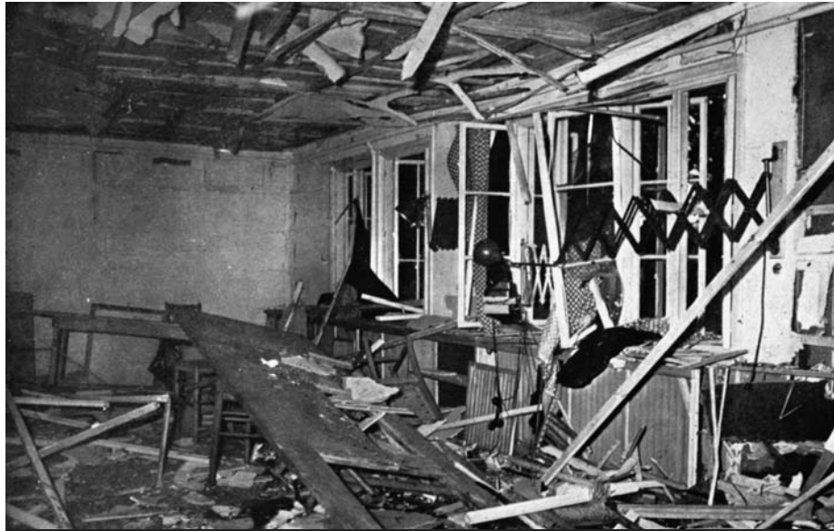
The shattered map hut where the explosive device was detonated on July 20, 1944, leaves little argument as to the fact that Stauffenberg believed Hitler was dead. An unwitting movement of Stauffenberg's briefcase by another officer is believed to have contributed to Hitler's survival.
