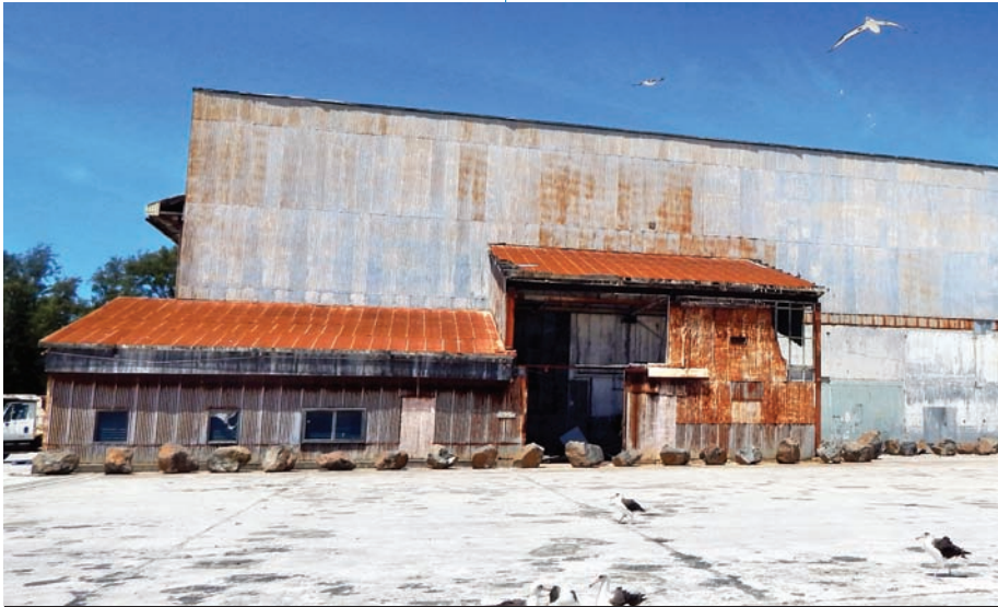
A 2015 photo of the ruins of the seaplane hangar on Midway Atoll. The building was heavily damaged during the bombardment of the atoll on December 7, 1941, when two Japanese destroyers unleashed a torrent of 5-inch shells.
