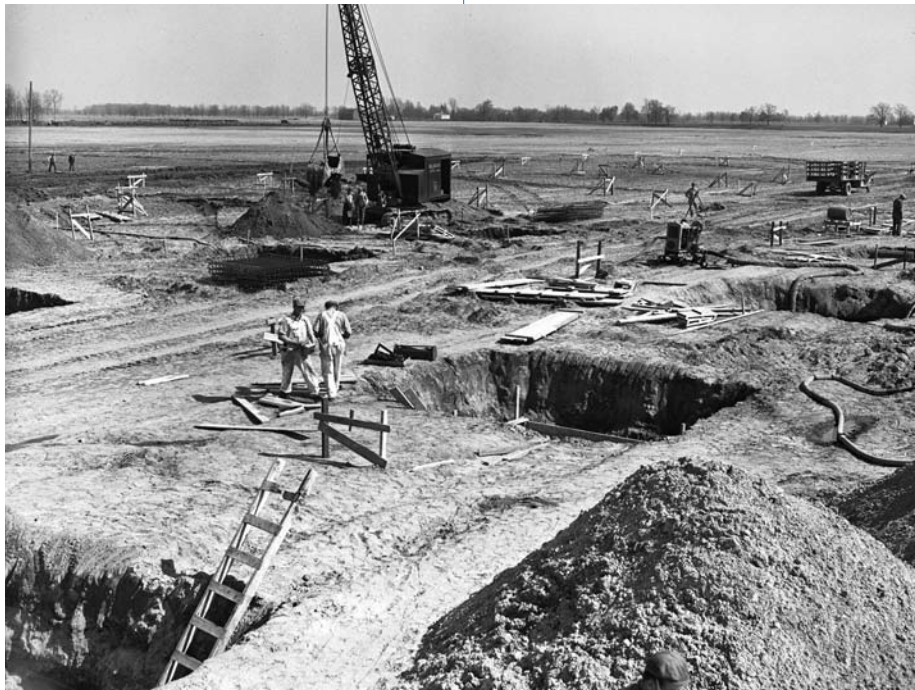
Willow Run plant under construction, 1940. With nearly 5 million square feet, the factory was touted as the largest single-story building in the world at the time.
