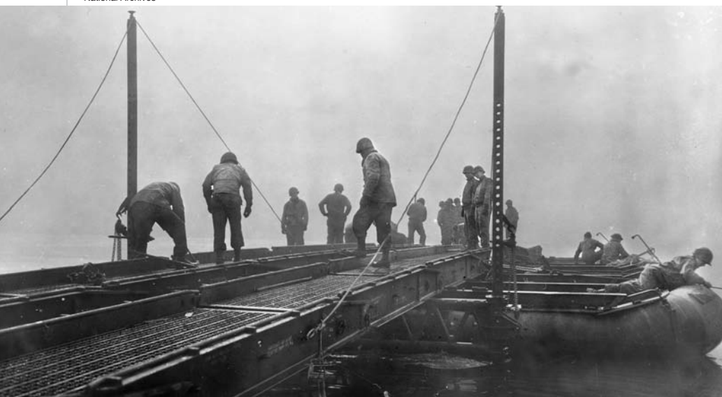
ABOVE: U.S. Army engineers attached to the 90th Infantry Division piece together a Treadway bridge across a German River. When a Messerschmitt fighter plane destroyed a bridge across the Werra River, Private Bernie Sevel found himself stranded on the far side. OPPOSITE: Two American soldiers scout past two German Hetzer tank destroyers. Much of Germany had been blasted to rubble by American air forces.
