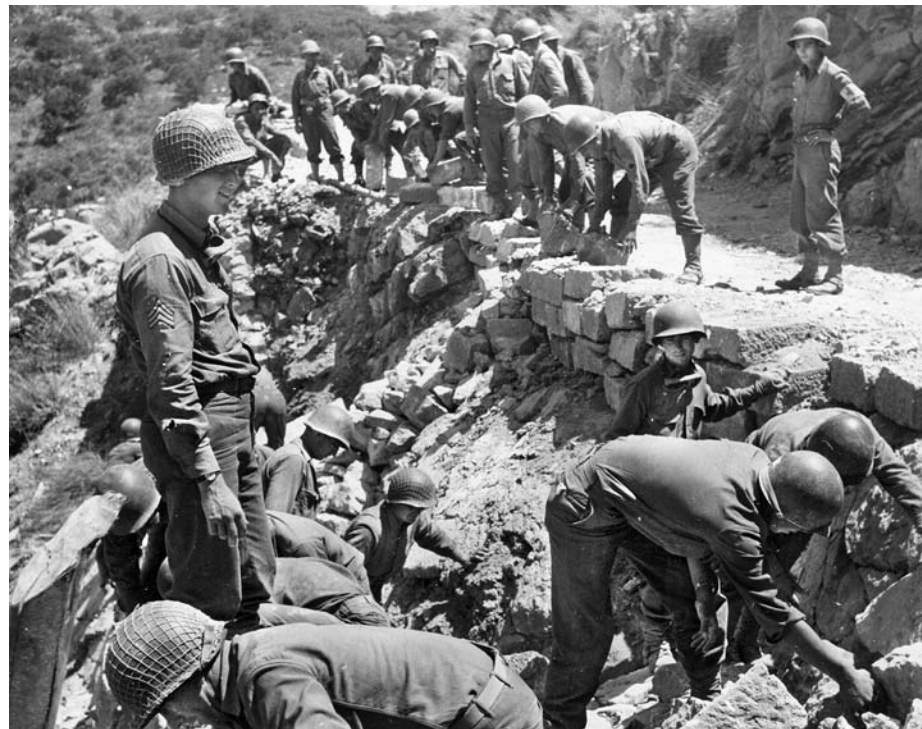
ABOVE: The Germans tried to slow the American advance from Palermo to Messina along the rugged northern coast of the island by destroying the roads. Here, American combat engineers work to repair the damage so the drive could continue. OPPOSITE: Urban fighting took place in Sicily's large cities and small villages. Here, men from the 6th Inniskillings, 38th Irish Brigade, 78th Battleaxe Division, search for enemy soldiers in a house during the battle for the town of Centuripe, August 2-4, 1943.
